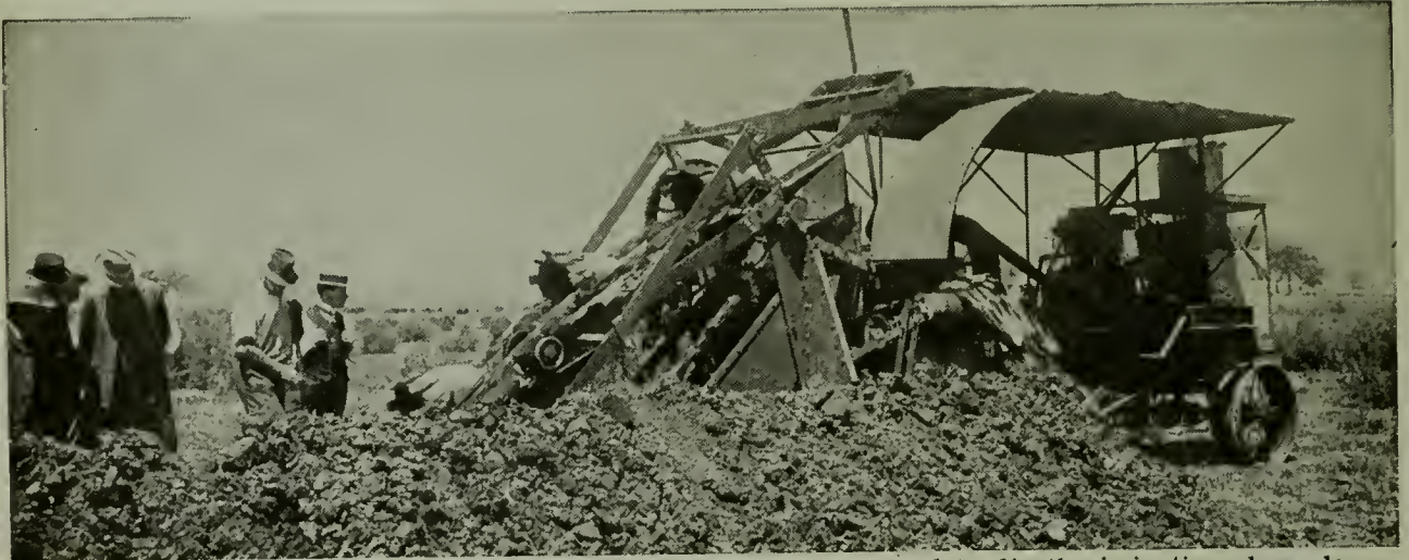
Where the ground is suitable, great mechanical excavators are used to dig the irrigation channels.
